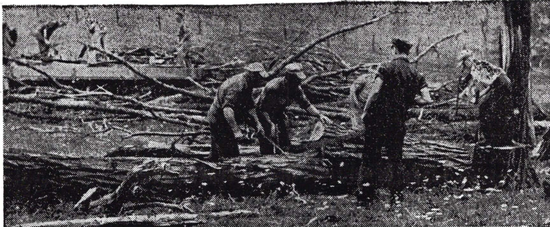
On the job bright and early and working up a good appetite are these men, shown cutting timber and cleaning up wind-tossed debris on the Moore farm. Clearing fallen timber was a tremendous task in all sections.
