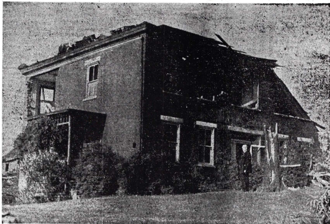
Pictured above is the large brick residence of Mr. and Mrs. William S. Lowry, one mile southwest of Independence, after it was hit by the devastating twister recently.
